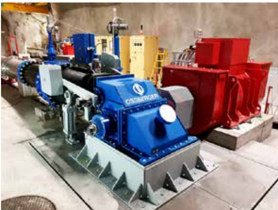
Residual water plant in Switzerland
